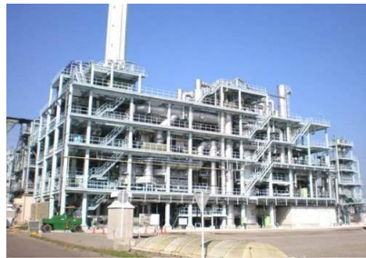
Sewage Sludge Carbonization Plant ①Bio Fuel Co.,Inc /Tokyo(Japan) ②2007③300t/d
