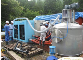
Mobile Siphon Tank
