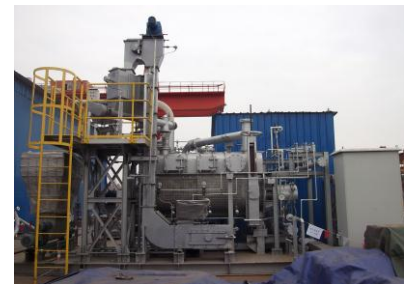
Sewage Sludge dryer ①China ②2012 ③15t/d
