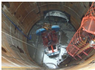
trunk line watershed manhole
