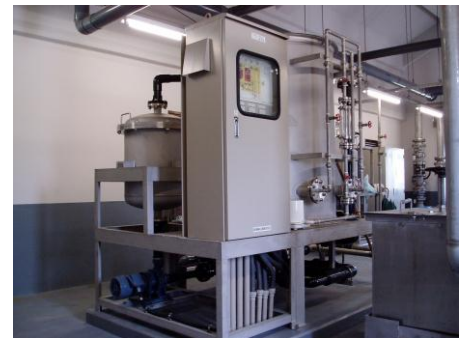
Sludge improvement/deodorizing equipment
